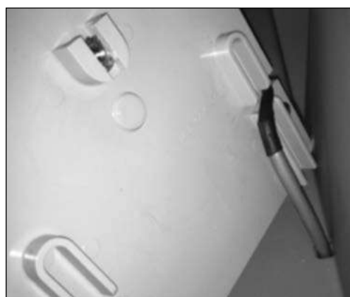
Figure 7.22 - Meter cable routed across back plate
