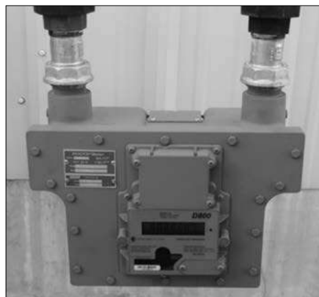
Figure 7.4 - Meter placed in line
